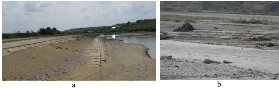
Fig. 7. General view of the Moldova River left bank in the groundwater catchment area a - shore protection structure (the old protection made of the slabs and the new one made of geo-bags); b - degradation state of the routing dike from the calibrated river bed right bank view (year 2018).
