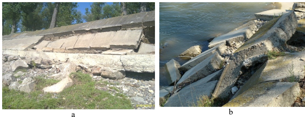
Figure 4: Degradation stages of Moldova River left shore protection: a - stone prism displacement, concrete slabs support beam breaking; b – slabs slipping on the embankment (2008).
